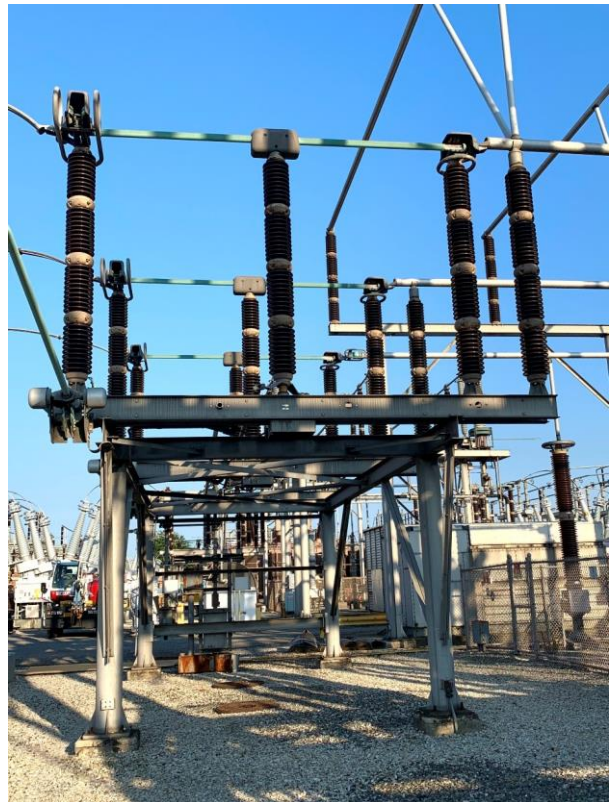
Figure 2: 345 kV Disconnect Switch w/Center-Pivot Horizontal Swing Arms
