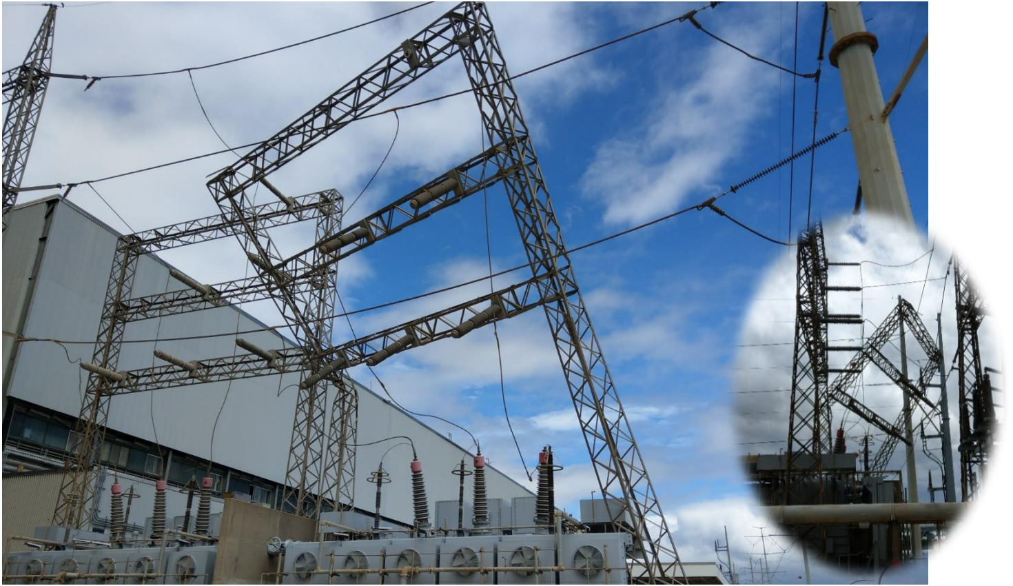
Figure 9.9: Damage at Substation
