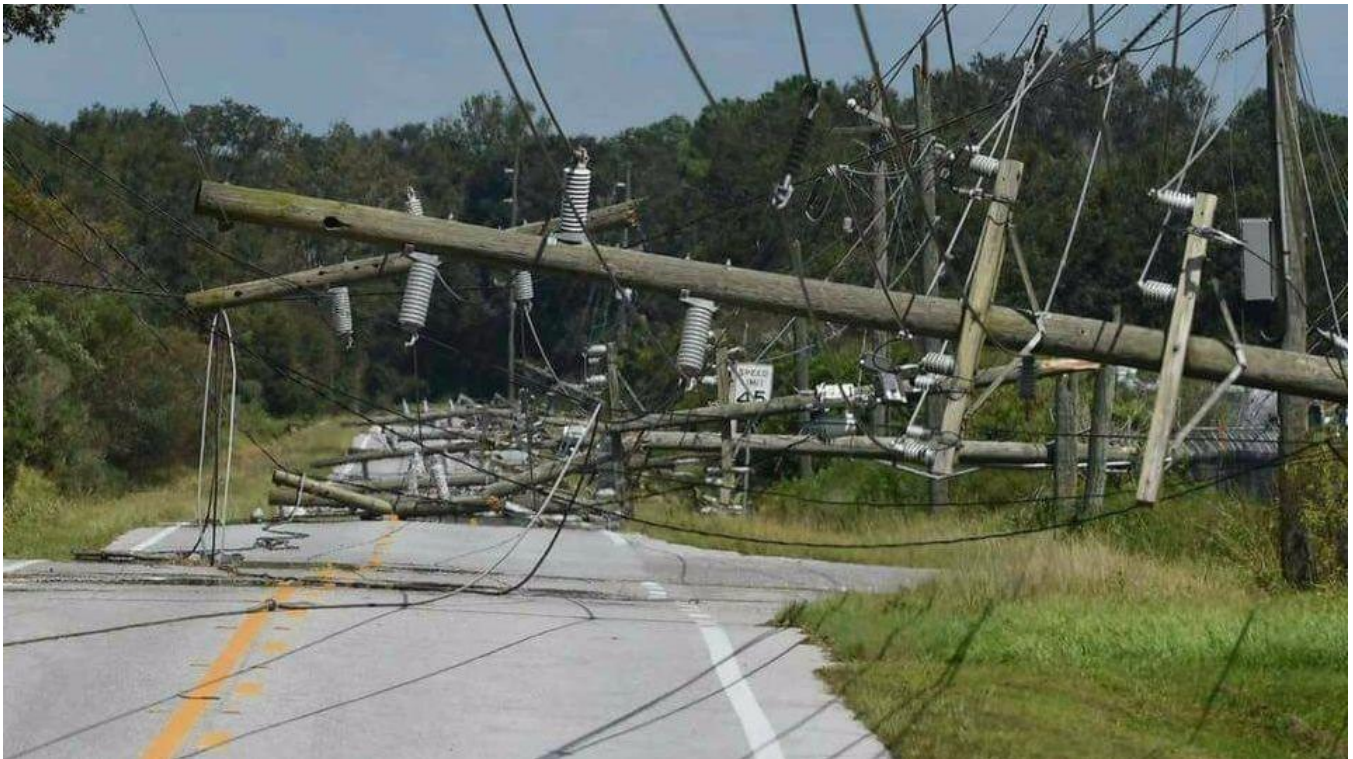
Figure 9.10: Damaged Transmission line with underbuilt distribution
