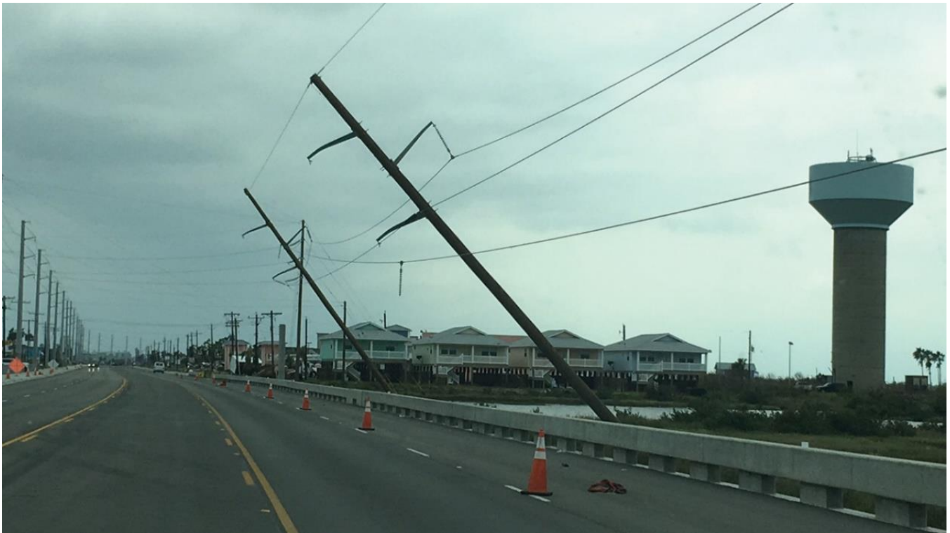
Figure 9.3: Example of damaged high voltage transmission line
