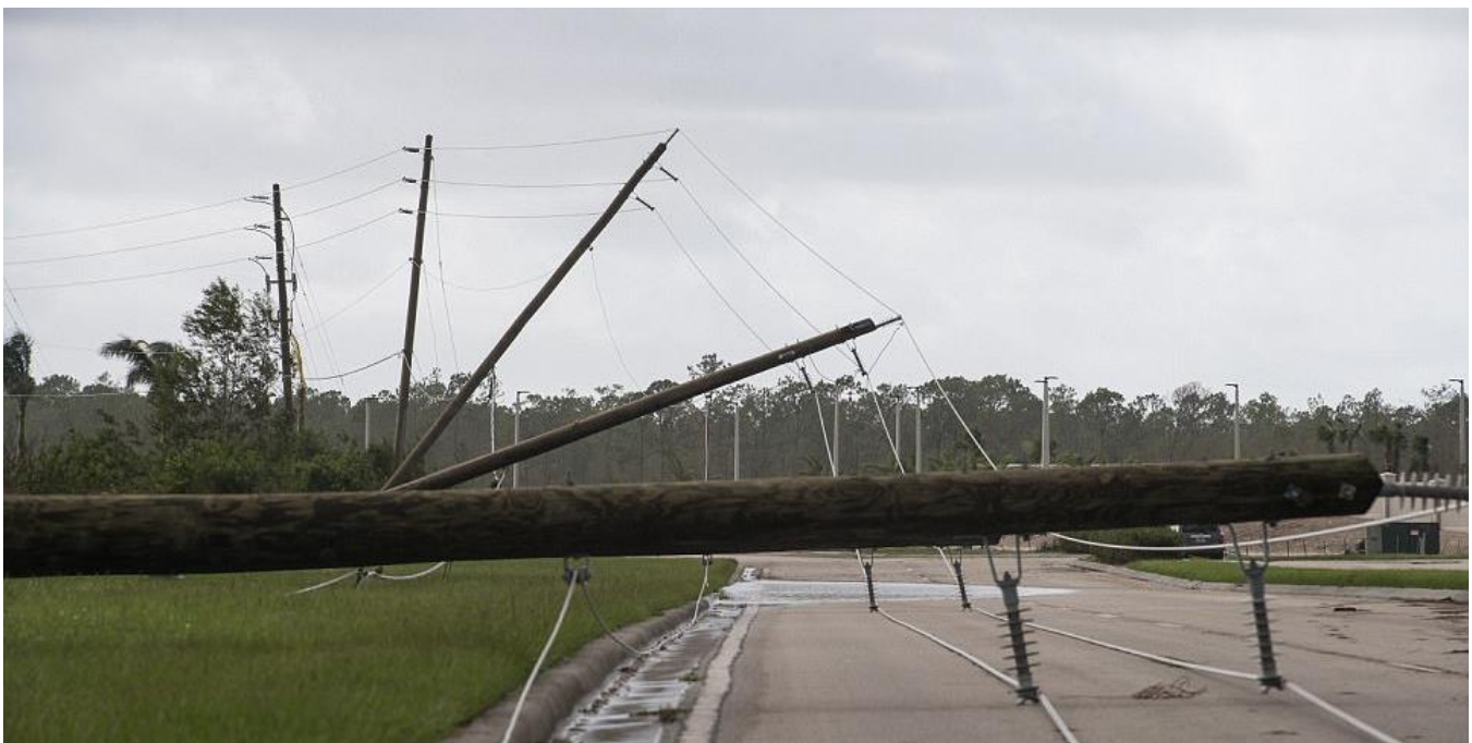
Figure 9.2: Example of damaged high voltage transmission line
