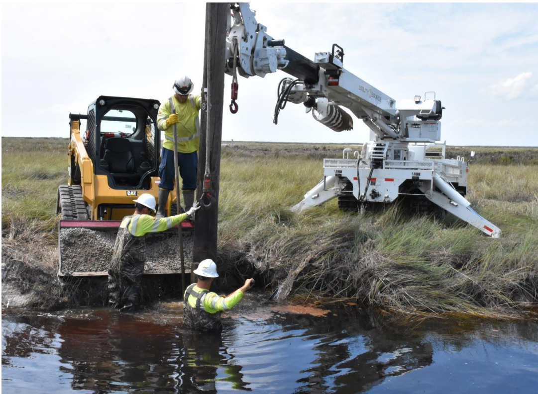
Figure 10.8: Flooding, mosquitos, as well as windy and muddy conditions created special challenges for work crews.
