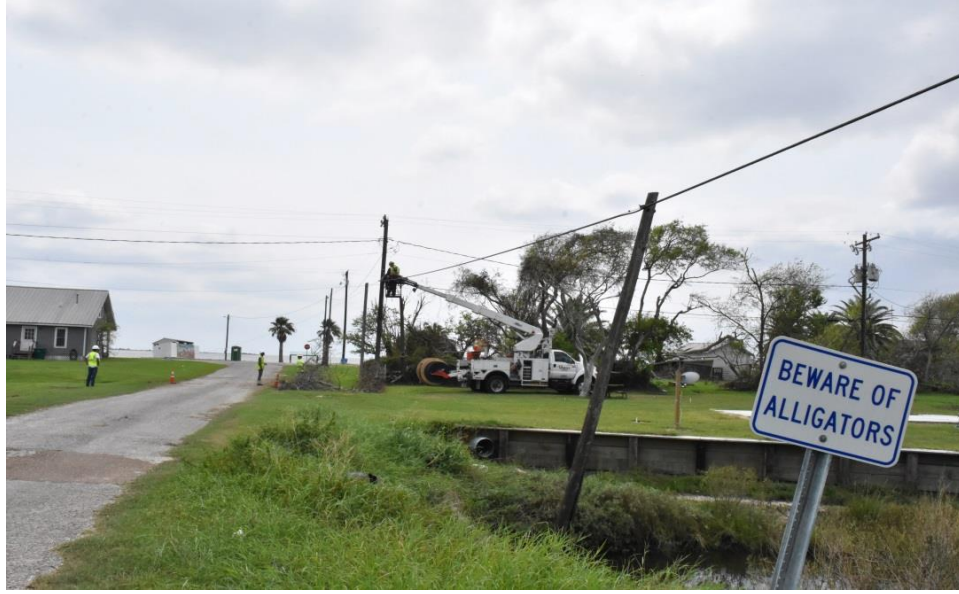
Figure 10.15: Examples of the damage sustained by the distribution system
