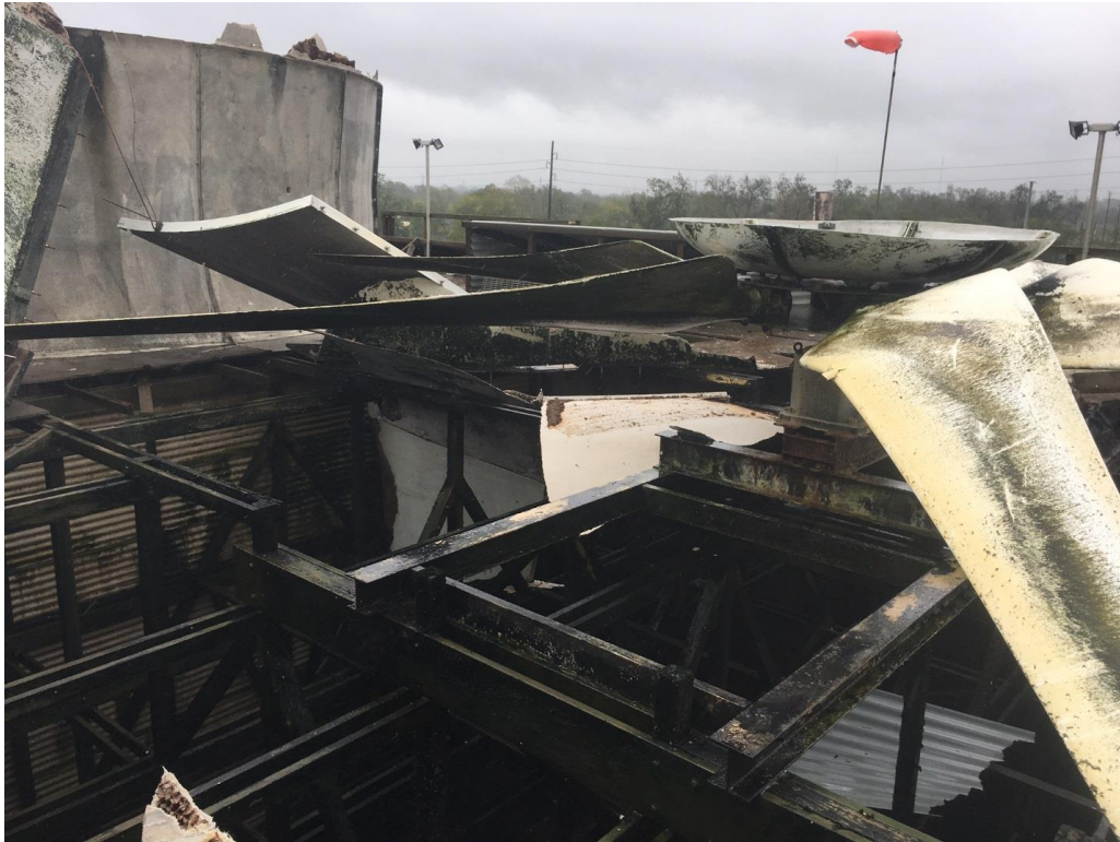
Figure 10.5: Damaged power plant cooling tower fan deck
