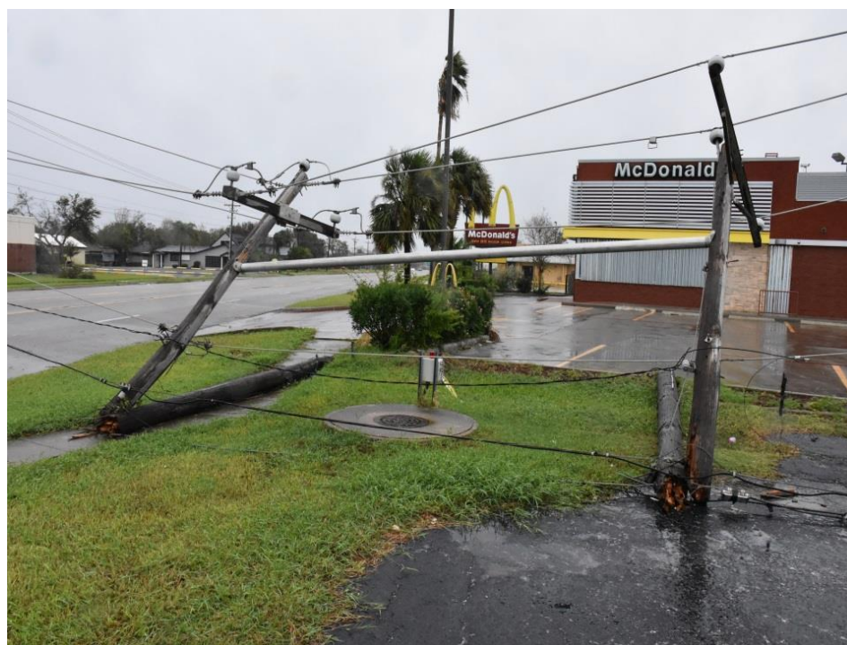
Figure 10.14: Examples of the damage sustained by the distribution system
