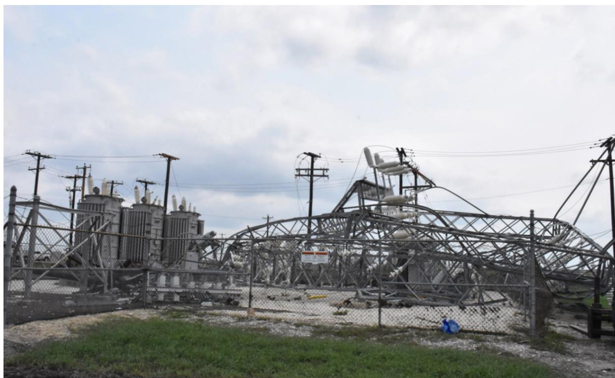
Figure 10.4: 69 kV substation structure damage
