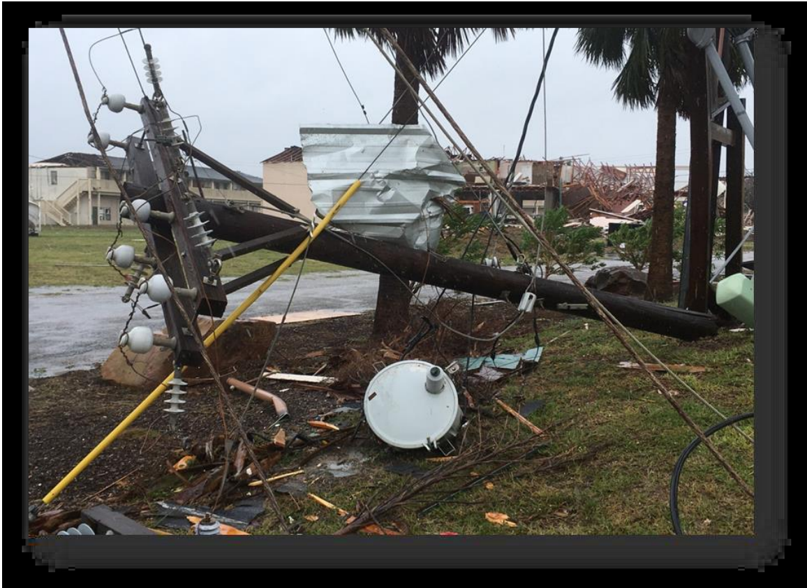
Figure 10.11: Examples of the damage sustained by the distribution system
