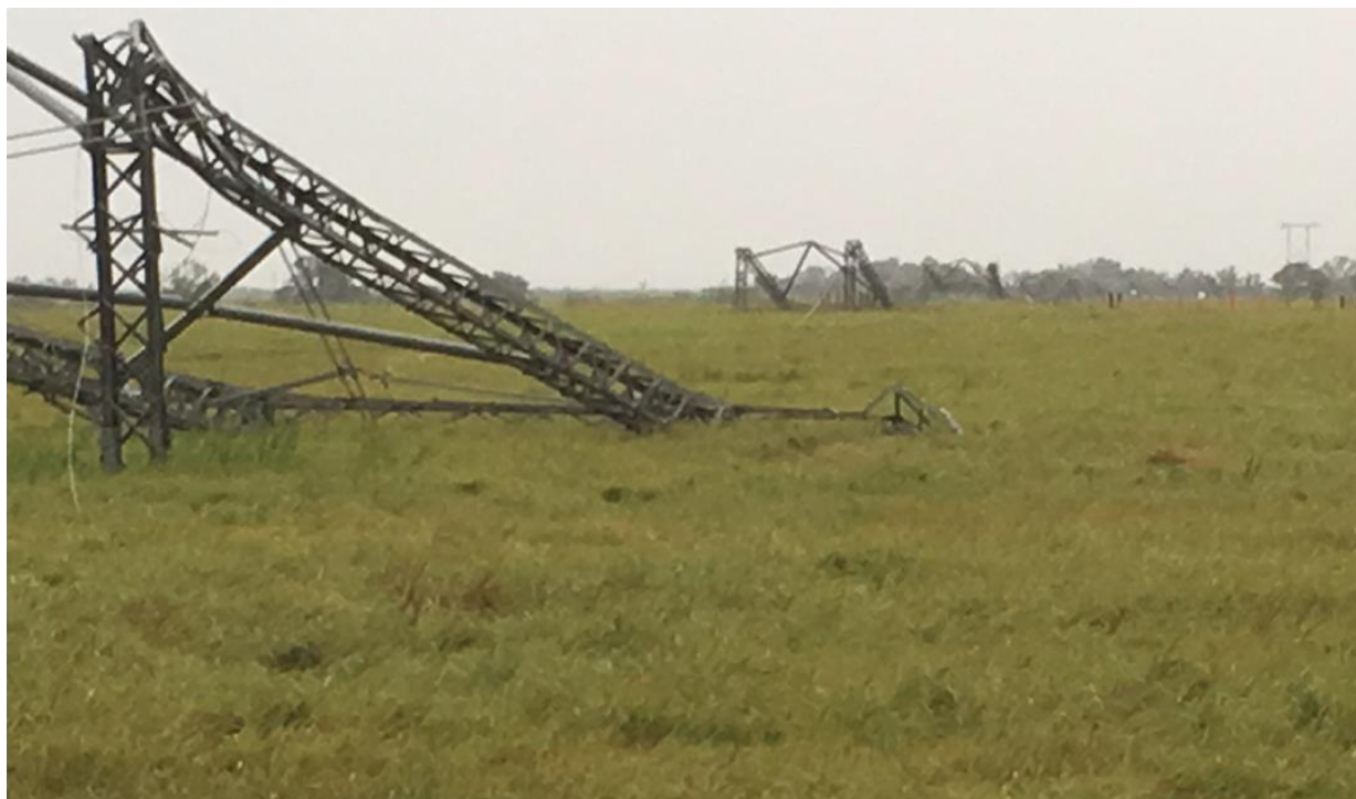
Figure 10.3: 345 kV line structures down
