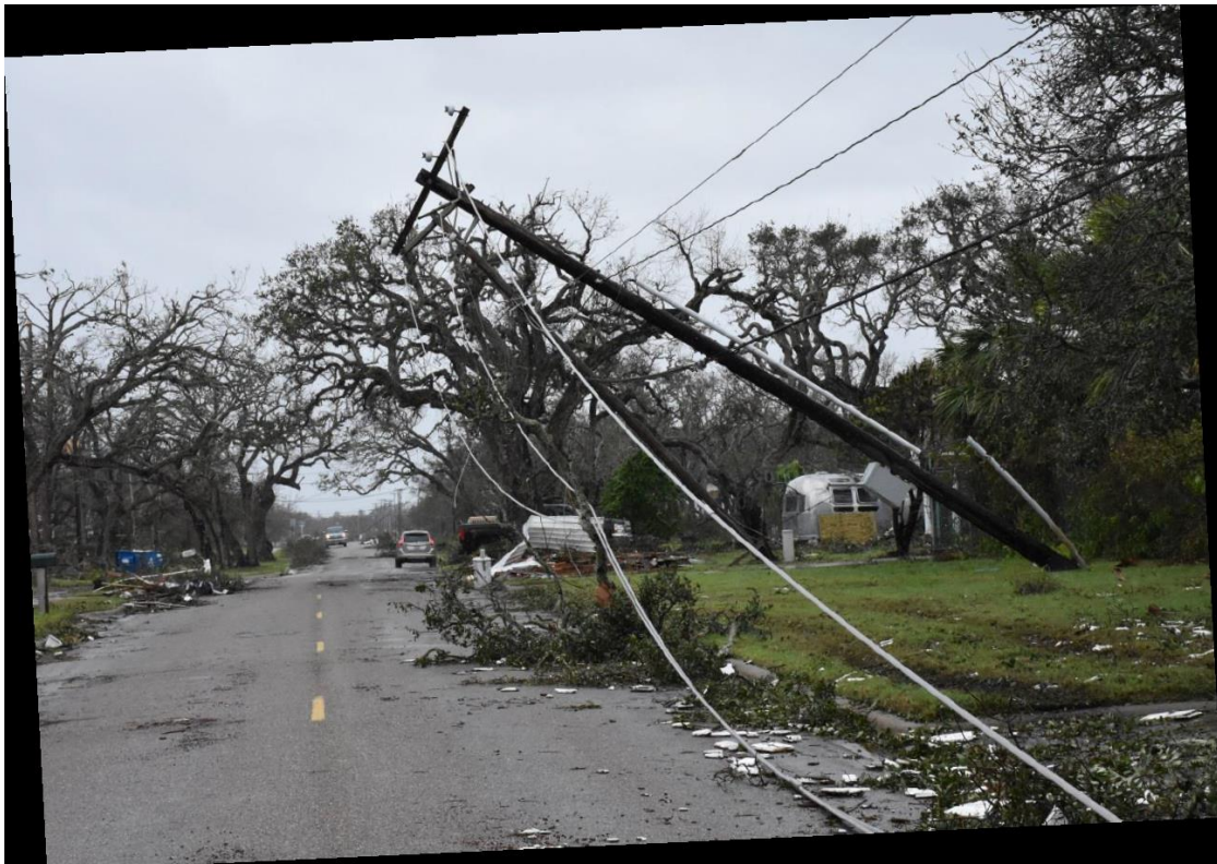
Figure 10.12: Examples of the damage sustained by the distribution system
