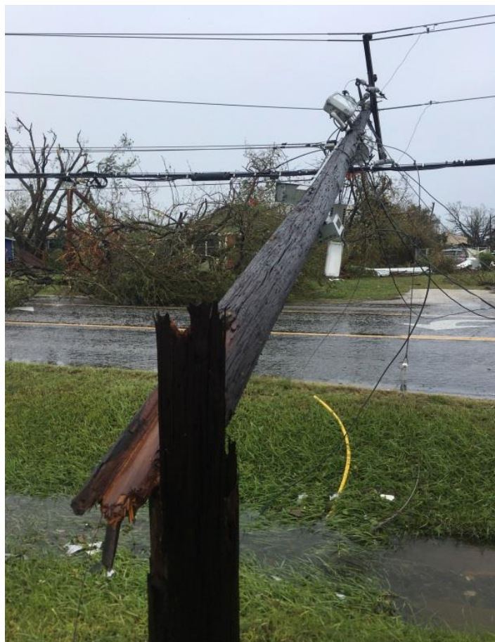
Figure 10.13: Examples of the damage sustained by the distribution system
