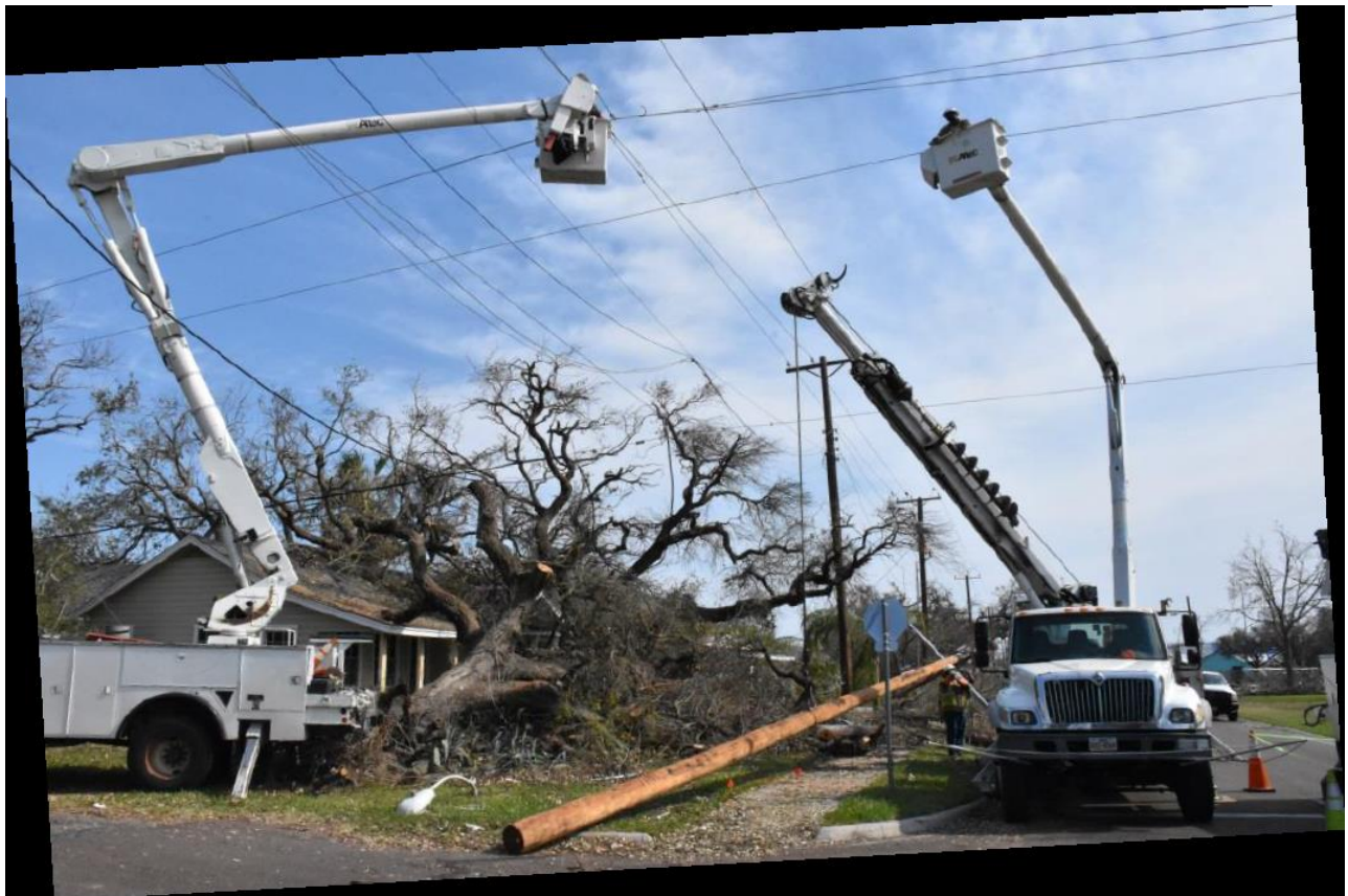
Figure 10.16: Examples of the damage sustained by the distribution system
