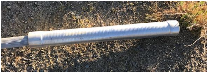
Figure 1.1: Photo of Failed Splice [Source: SCE]
