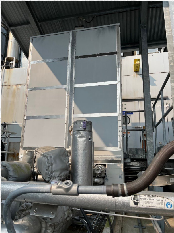
Water injection Skid
