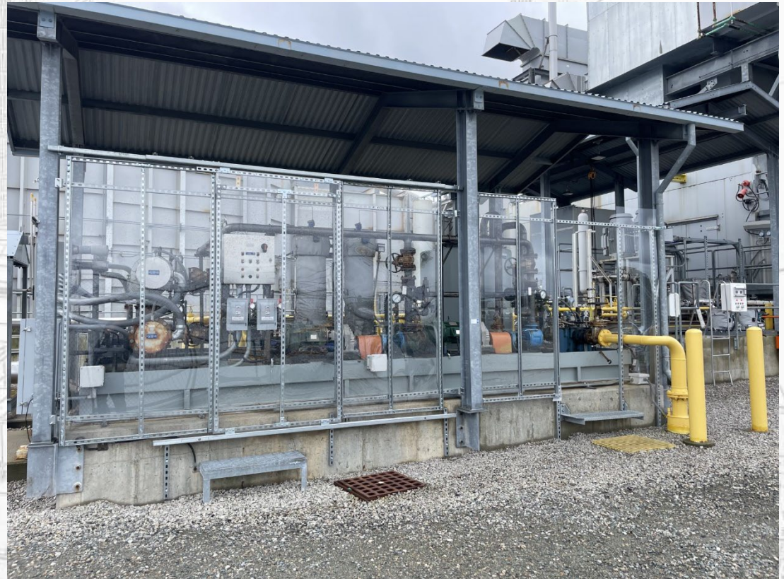
Low Pressure Fuel Oil Skid Strategic Sliding Plexiglass panels
