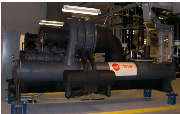
Figure 8: Large Three-Phase (Chiller) Induction Motor Example
